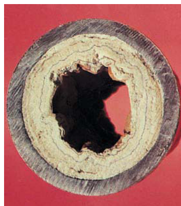
FIGURE 11.8 A pipe with accumulated mineral deposits. The cross section clearly indicates the reduction in pipe capacity.
